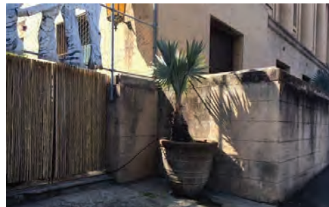
Figure 47: Stone retaining wall on the north-west corner of the building (Source: NBR SARCHITECTURE 2018)
