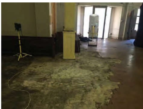
Figure 58: Parquet flooring, showing damaged section, on the lower ground floor (Source: NBR SARCHITECTURE 2018)
