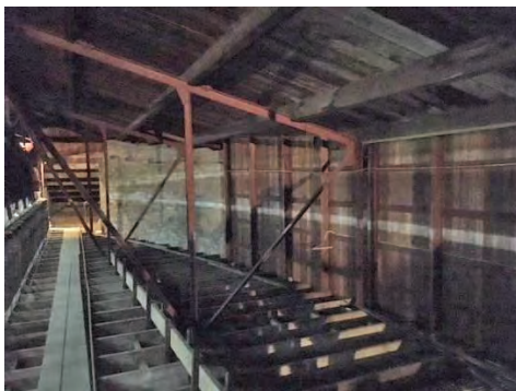
Figure 88: Roof space above the organ, to the west of the organ chamber (Source: NBR SARCHITECTURE 2018)
