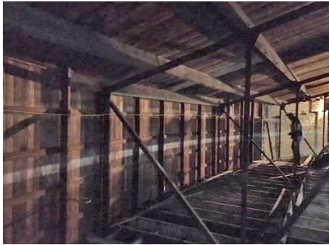
Figure 86: Perimeter roof space on the southern side of the building (Source: NBR SARCHITECTURE 2018)
