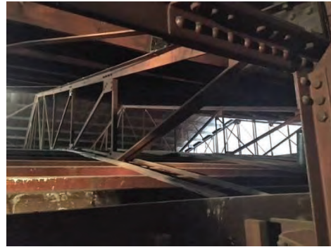
Figure 87: Roof space above the auditorium, showing its curved structure and steel trusses (Source: NBR SARCHITECTURE 2018)
