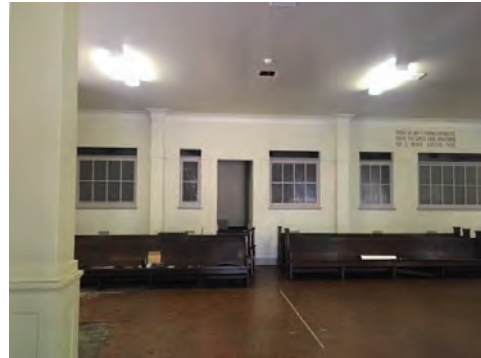
Figure 57: Rear rooms to the former Sunday School, facing east (Source: NBR SARCHITECTURE 2018)
